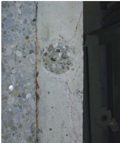
Fig. 4 Punch cone of a dismantled test specimen
